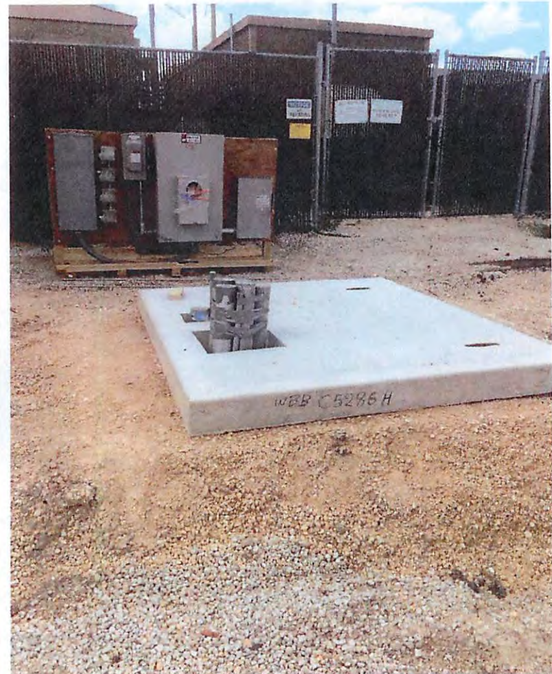
Transformer Pad & Temporary Gear
