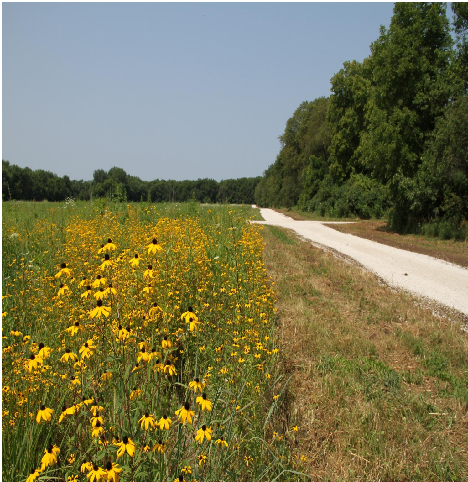
Genoa to Russell Woods trail under construction (Russell Woods in far background, Genoa Prairie in foreground)
