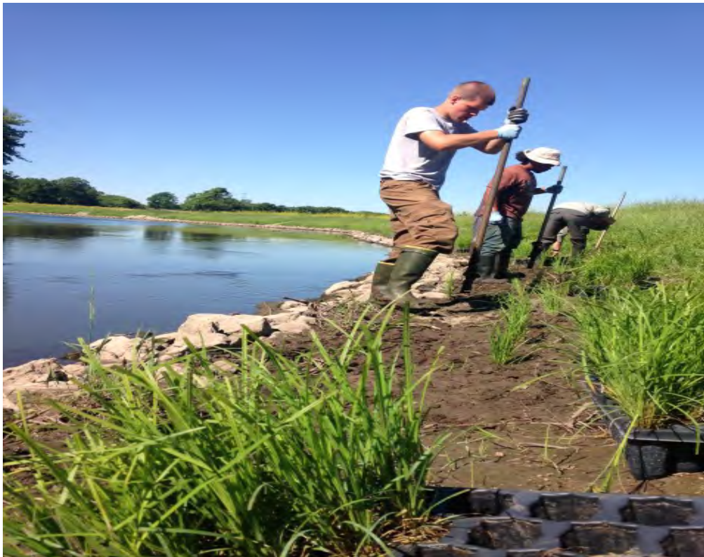
Interns plant sedges along the Kishwaukee River at the streambank stabilization site.
