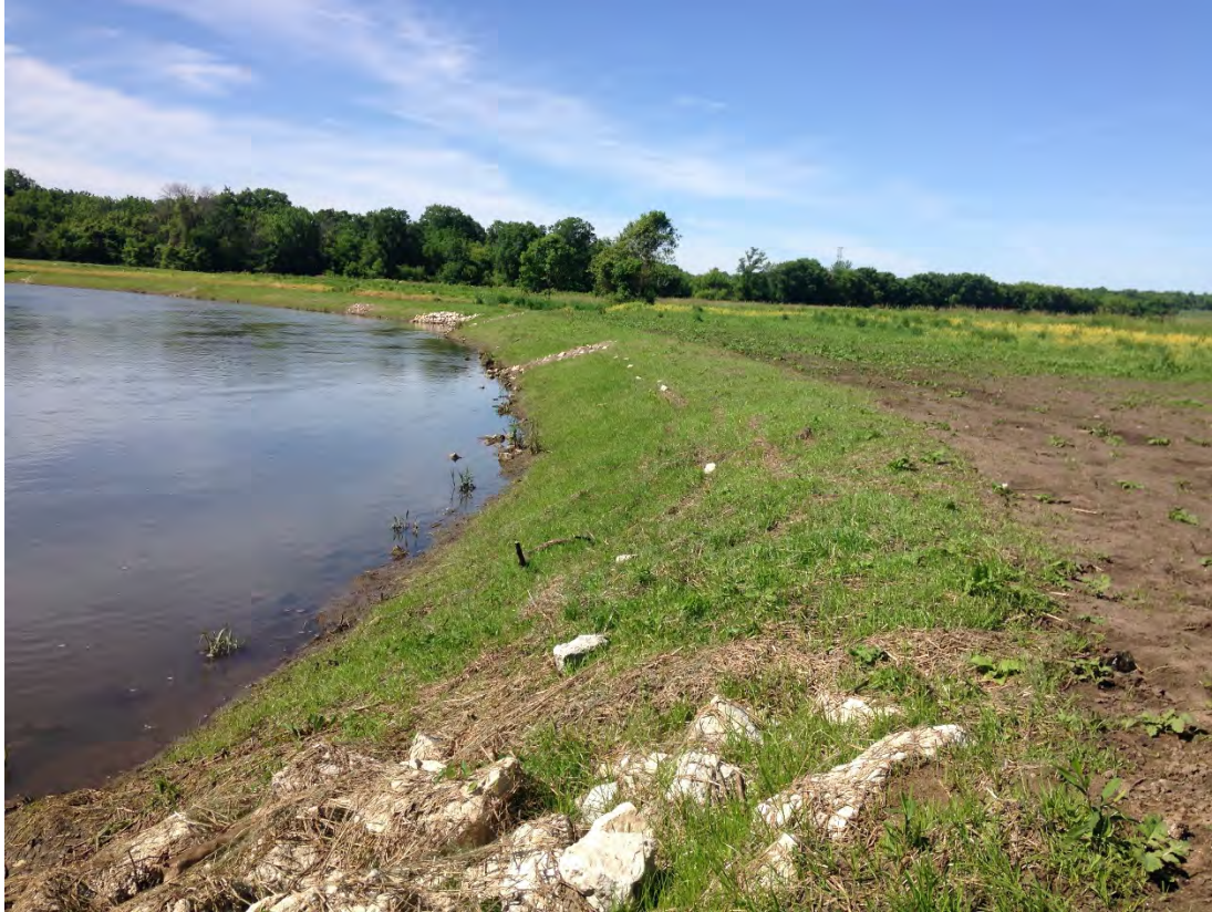
The streambank stabilization at the Kishwaukee River project in the South Branch Prairie is stable and greening up despite the high water and flooding all month long.
