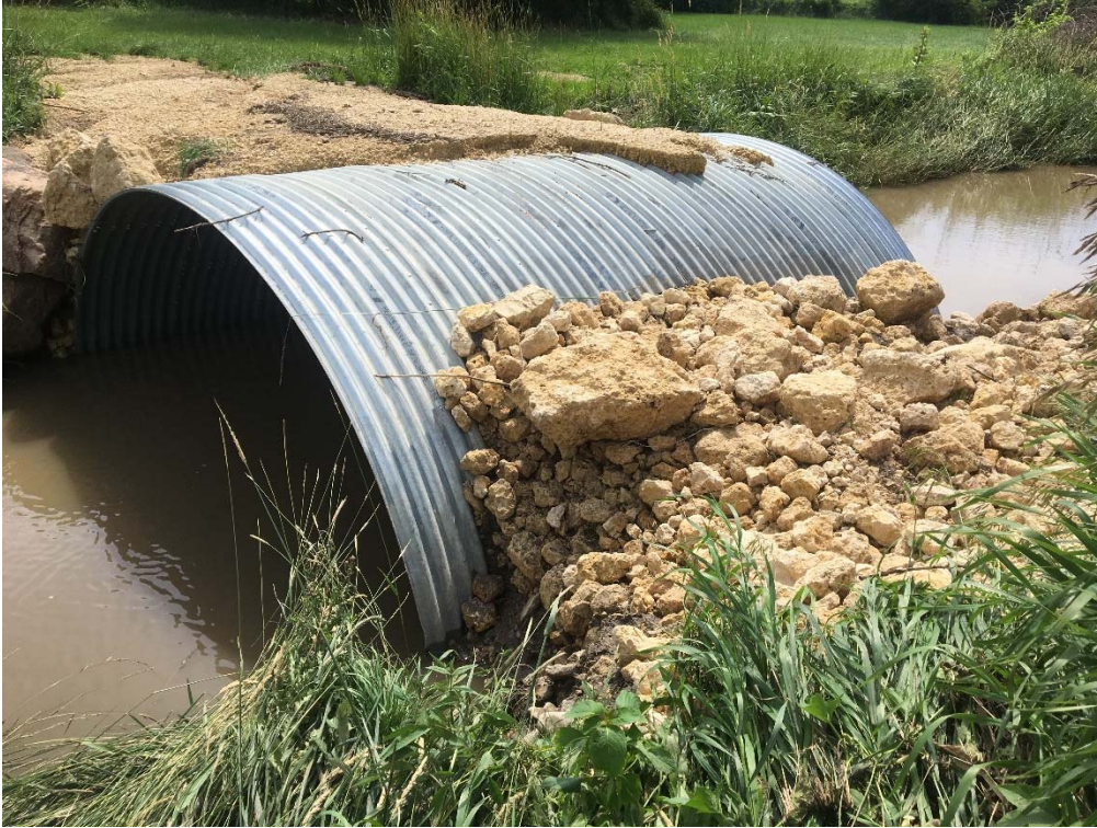
The impact of heavy rains on the access lanes at the new Swanson Grove site.
